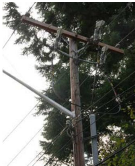
Typical 3-phase distribution underground termination (cables rising up to connect to overhead lines)
