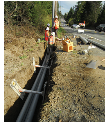
Underground distribution cable in a trench in Fairwood, WA
